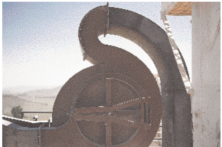
The limestone facility's centrifugal air classifier sizes limestone dust to -325 mesh.
